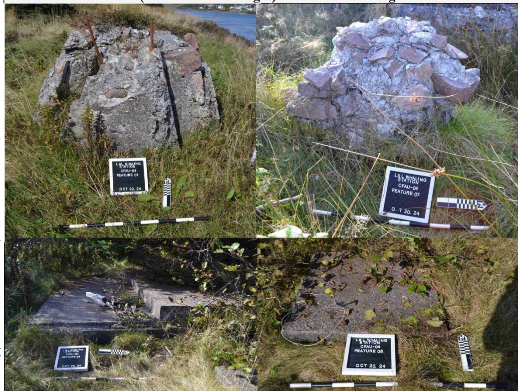
Figure 5: (Top Left and Right) Badly deteriorated concrete blocks. (Bottom Left and Right) Concrete blocks in good condition.
