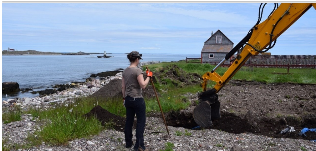
Figure 1: Field Director, Catherine Losier, closely monitoring the backhoe removing sod and emptying out Sector 5 which was excavated during the previous season
